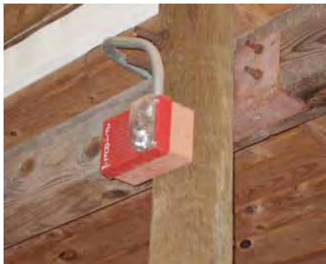
Fig. 6. Fire alarm siren and visual strobe light in conduit in a barn. Photo courtesy of Tomas Gimenez.
