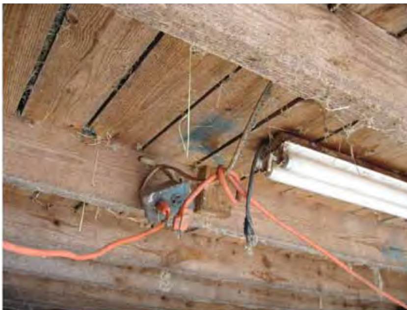
Fig. 14. Poorly designed and managed electrical service in a 12-stall horse barn. Photo courtesy of Tomas Gimenez.
