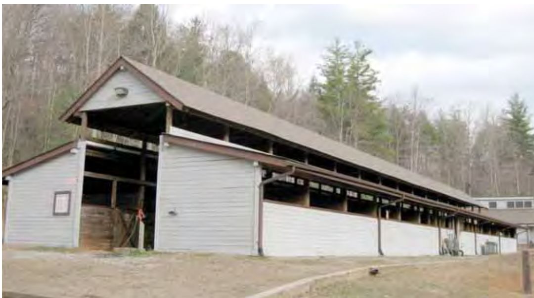
Fig. 16. Public horse barn built with fire safety in mind: open ventilation, frost-free hydrants, and 33 m of defensible space around the structure. Photo courtesy of Tomas Gimenez.
